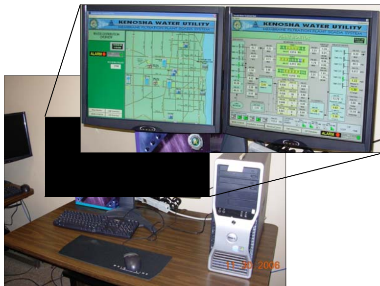
New Workstation with Double Monitor Installed
