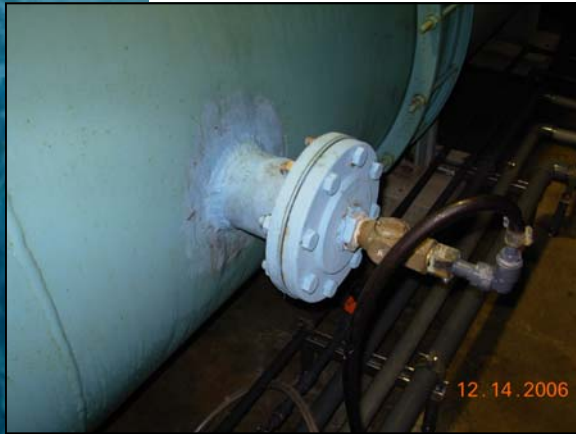
Chemical Feed Pipe Before Repair
