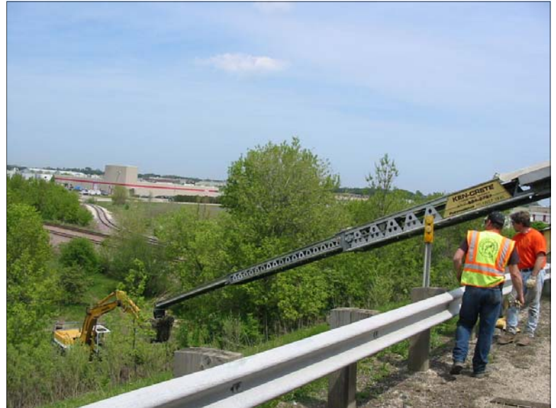
Water Utility employees look on as backfill material is being lowered down the embankment.
