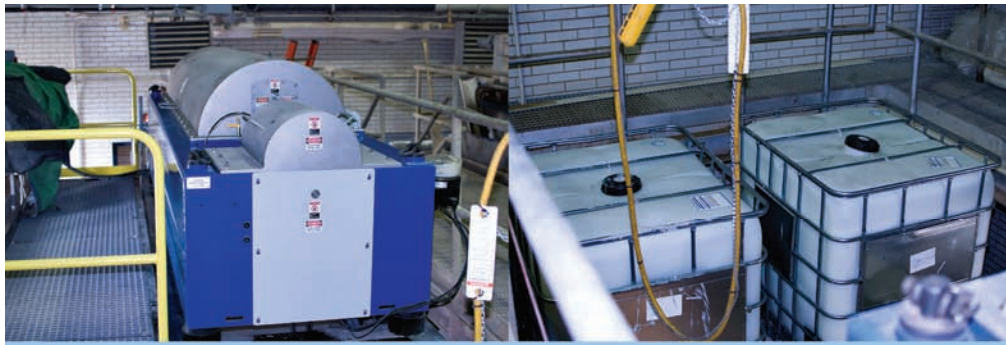
1. Newly installed centrifuge in operation dewatering sludge.
